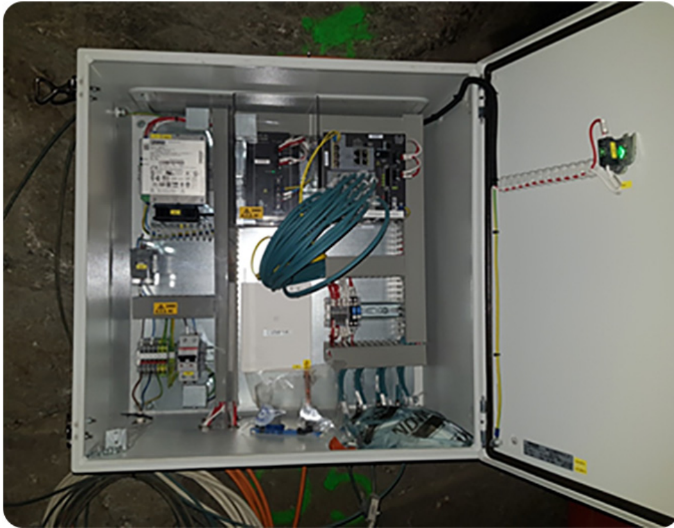
Figure 78 Pre- Fabricated Mine Enclosure for Cisco IE switch and components
